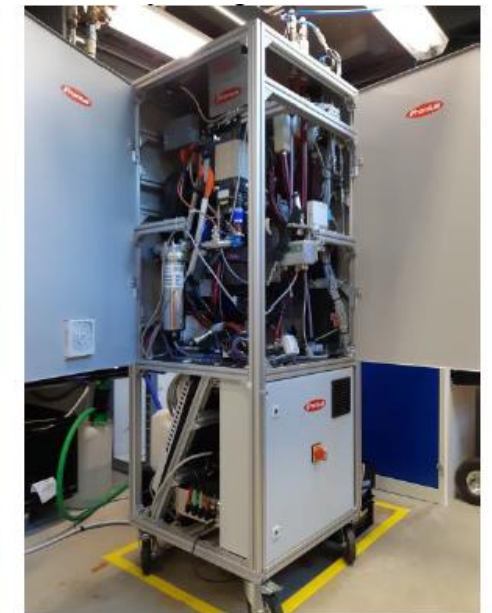
Fuel Cell System
